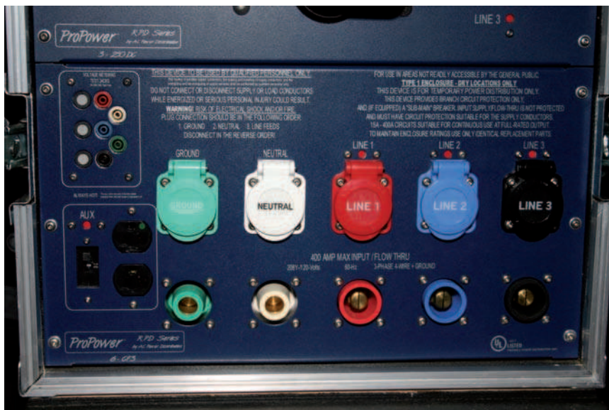
Figure 6-18 120/208 VAC four-wire plus ground electrical distribution panel.
