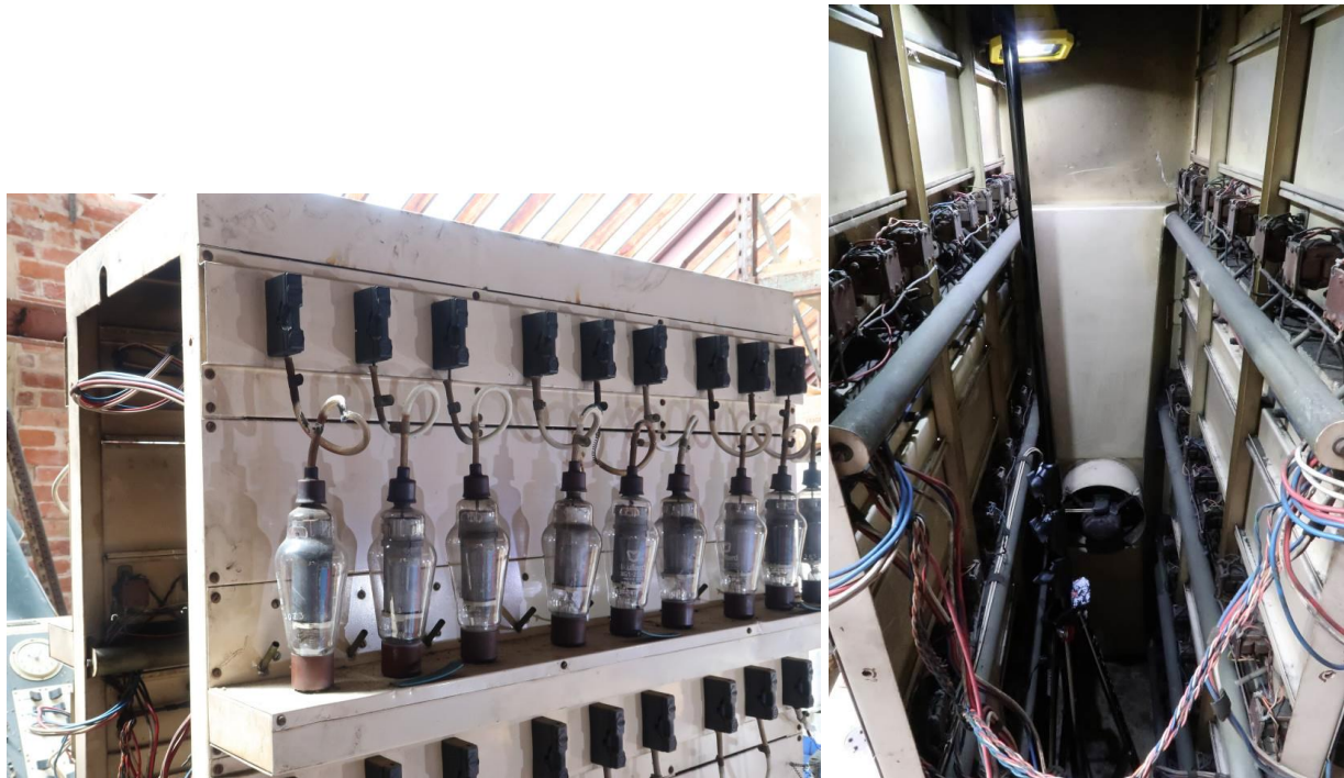
Figure 20. (left) View outside and (right) inside Manchester valve rack from centre
