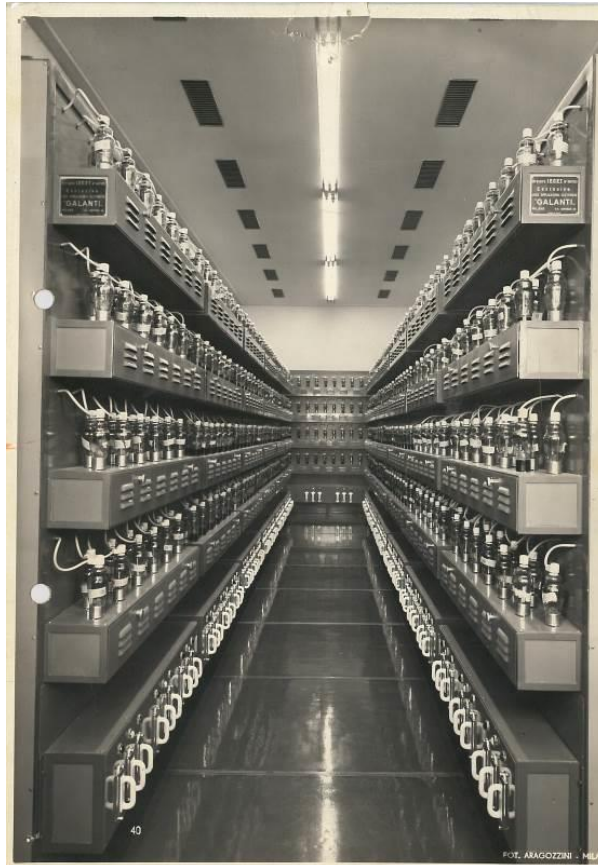
Figure 53. Italian ‘Galanti’ thyatron dimmer racks, probably at La Scala, Milan (Brown 1953-56).
