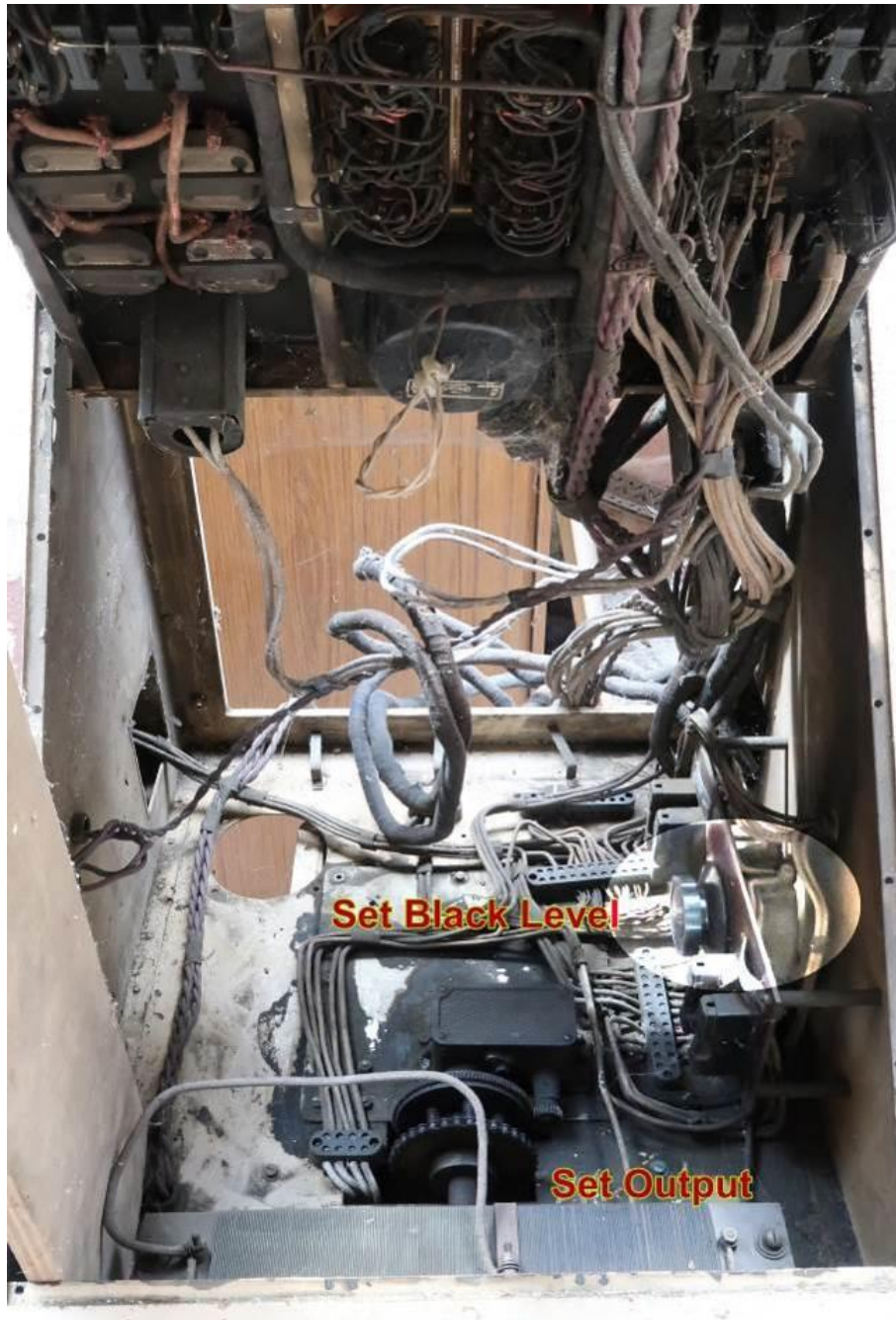
Figure 27. Interior of master panel with setup adjustments
