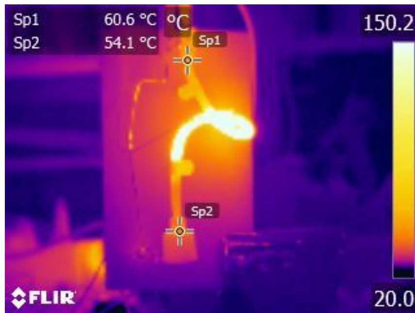
Figure 22. IR image of anode lead carrying 4.81 A rms
