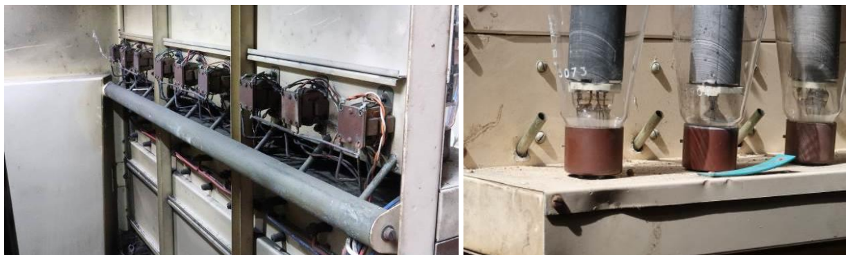
Figure 21. (left) Rear of valve rail showing grid transformers and (right) cooling ducts to valve bases
